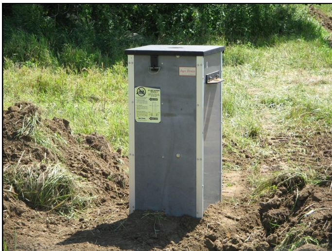
Tile Management Structure—reduces nitrogen loss by lowering the amount of total outflow, primarily during the winter.
